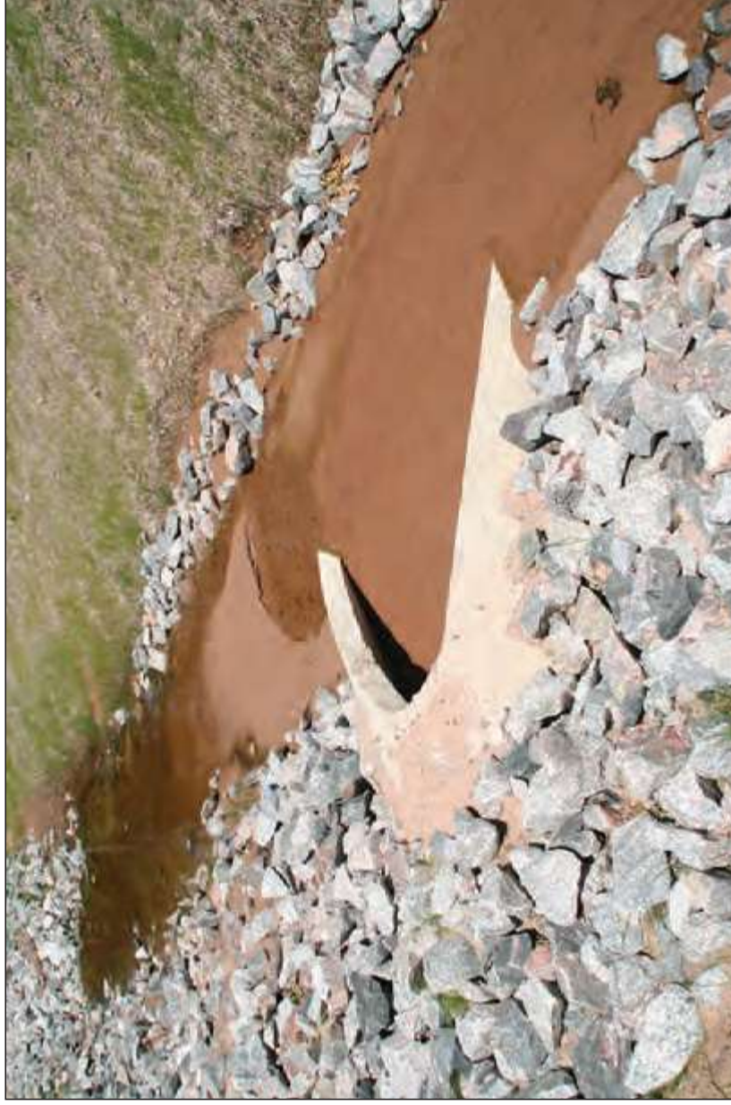
Undersized sedimentation basin along a mine haul road. The sediment will need to be removed for the basin to work as intended.
